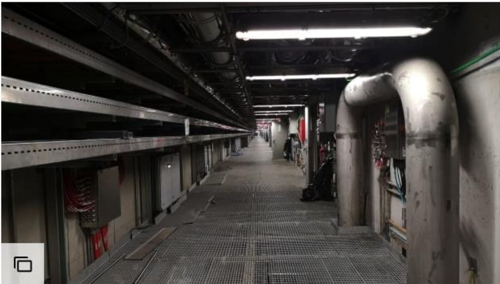
The underwater tunnel follows the barrier from Punta Sabbioni to the Lido.
